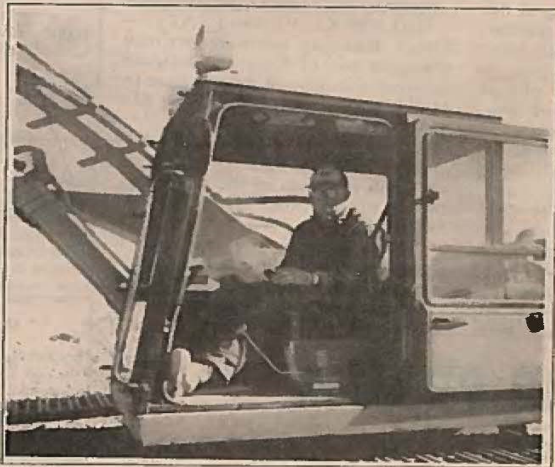
Jerry Robison is volunteering his time to operate Mike Lemich's track backhoe to cut trenches for the heat system at Great Basin College.
