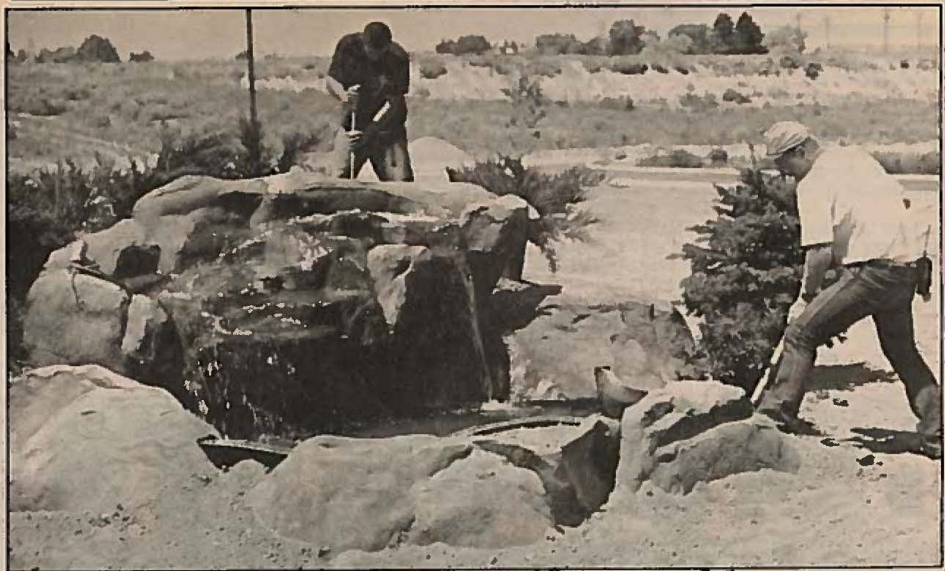
Fountain: Clyde Gregory, left, and Todd Shouse of Kimberly Nurseries are putting the finishing touches on the fountain outside Northern Nevada Community College Foundation's new theater, scheduled for completion at the end of the month. The foundation is already planning its Oct. 21 dinner/
