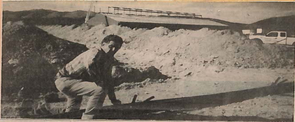
Jim Lewis unloads ground-source heat pipe at Great Basin College. He is providing technical guidance and hands-on supervision over the project.
