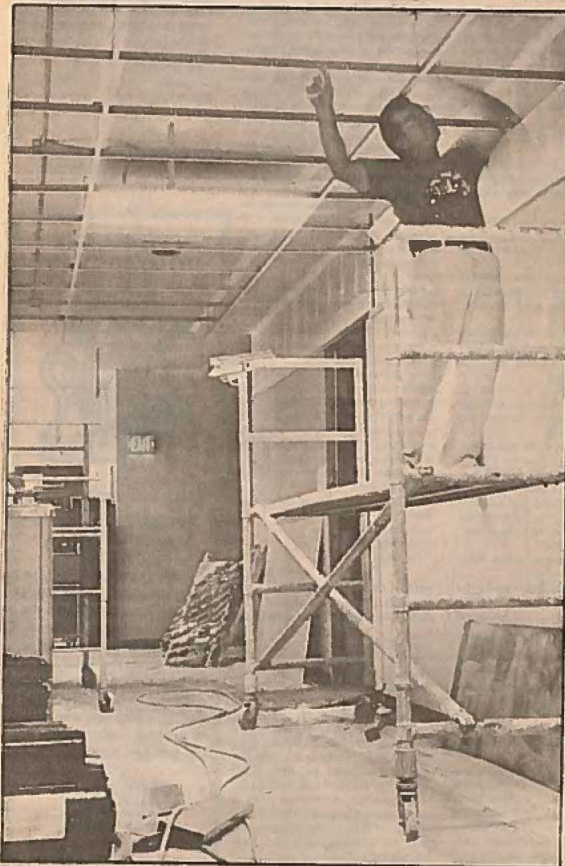
Worker Frank Evans of Tahoe City, Calif., tapes off newly installed ceiling supports. Remodeling has included putting a lower ceiling into the building. Work is expected to be finished in about two weeks.
