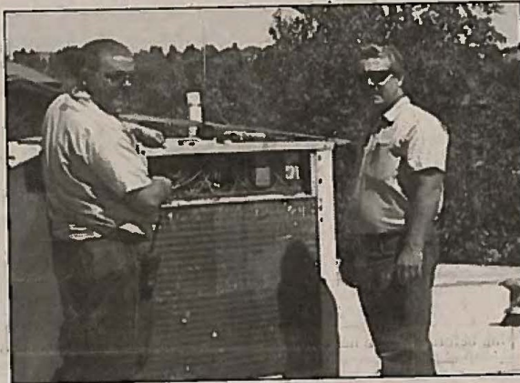
JENNIFER SIMONSEN • Winnemucca News Service Electrician Rocky Dunham (left) and heating specialist Steve Ricords work on Great Basin College's Elizabeth Griswold Hall rooftop to oversee the building equipment before new students move into the dorm.
