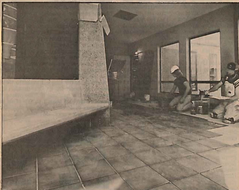
The exterior of Northern Nevada Community College's Phase III building (top photo) is basically finished. The new structure is located in the northwest section of the campus. In lower photo, Andy Ketterer (left) and Brent Barney wrapped up the tile work in the Phase III lobby Wednesday. Both workers are from Wasatch Tile in Salt Lake City. Additional photos appear on Page 3.
